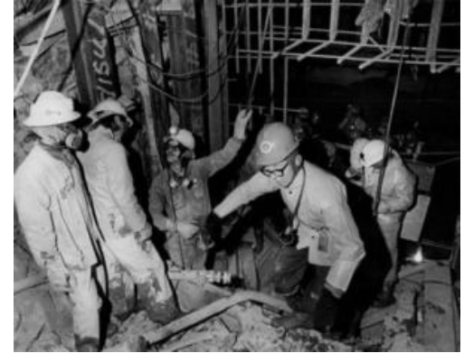
The Lady Is A Miner - Janet Bonnema (right) makes her way through the Straight Creek Tunnel. Miss Bonnema, 33, of Georgetown, Colorado, had been hired to work in the tunnel a year and a half ago, but was sent to the division office instead of working in the tunnel. Janet filed a suit, charging sex discrimination against the Colorado Division of I Highways. Miss Bonnema was assigned as a rock mechanic, a Job which requires periodic trips into the tunnel. Shouting, "Get the women out of here," about 60 workers walked off the job. (Photo By Duane Howell/The Denver Post via Getty Images)
